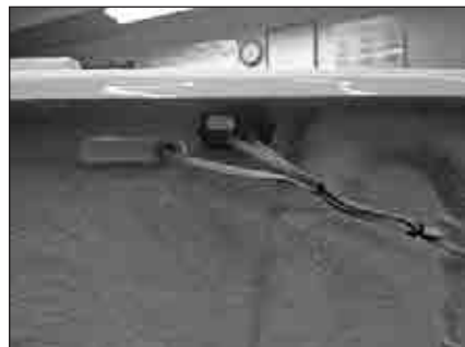
Modules and keypads are factory installed
